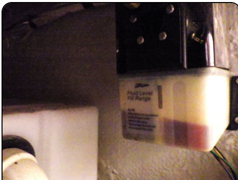
Trim tab reservoir was observed to be low
